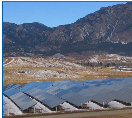
Solar panels at Fort Carson
